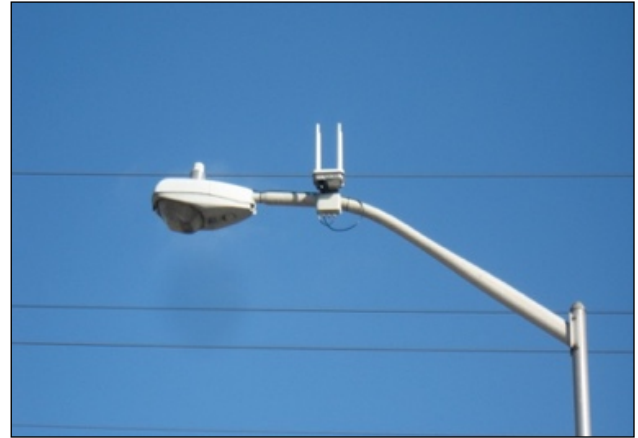
Figure 3 WiFi transceiver mounted on Lamp post
